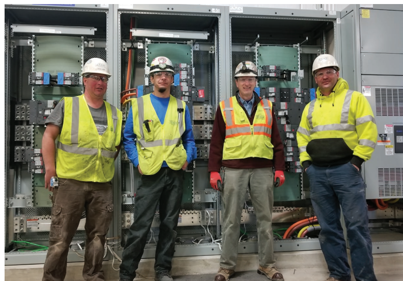
Pictured below (L to R): Egan Electricians Dan Weber, Kristopher Durand, Dennis Belanger, and Derrick Frank
